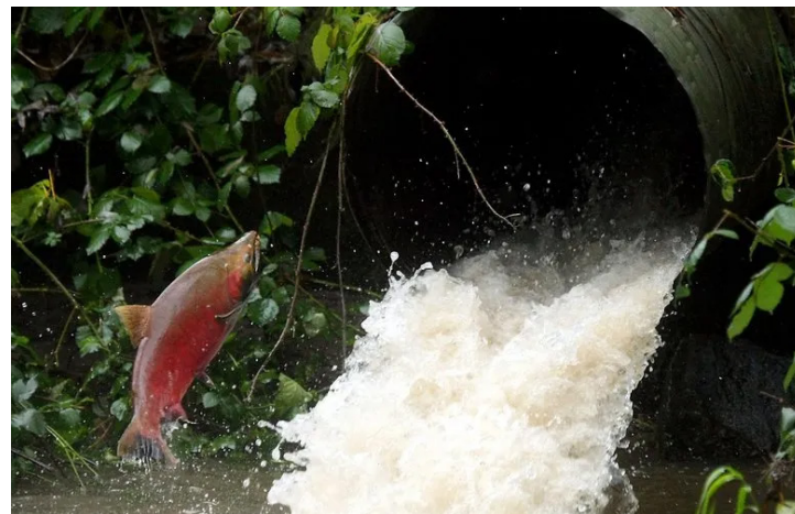
Figure 19. Salmon attempting migration up an undersized, perched culvert. Source: Meegan M. Reid/Kitsap Sun via AP, 2019)
