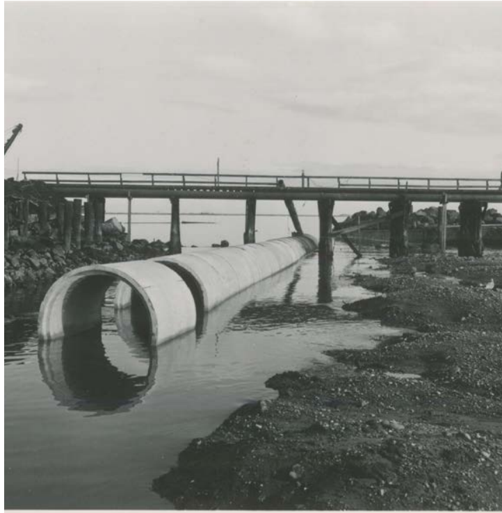
Figure 58. Valley Creek culvert installation, 1957 Source: Photo courtesy of North Olympic History Center, 2023
