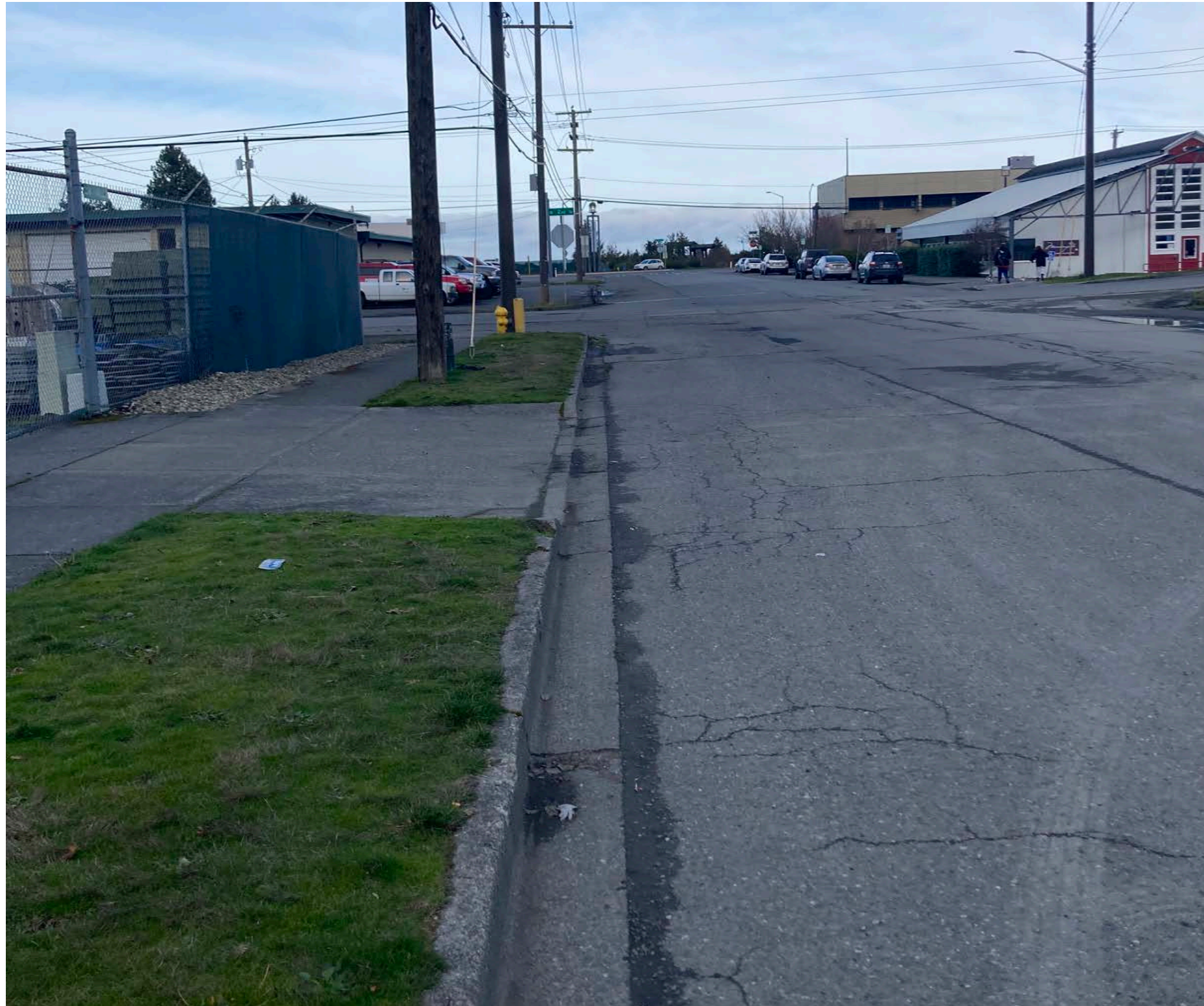
Figure 7. View looking north on South Valley Street, where the roadway overlays the Valley Creek culvert system
