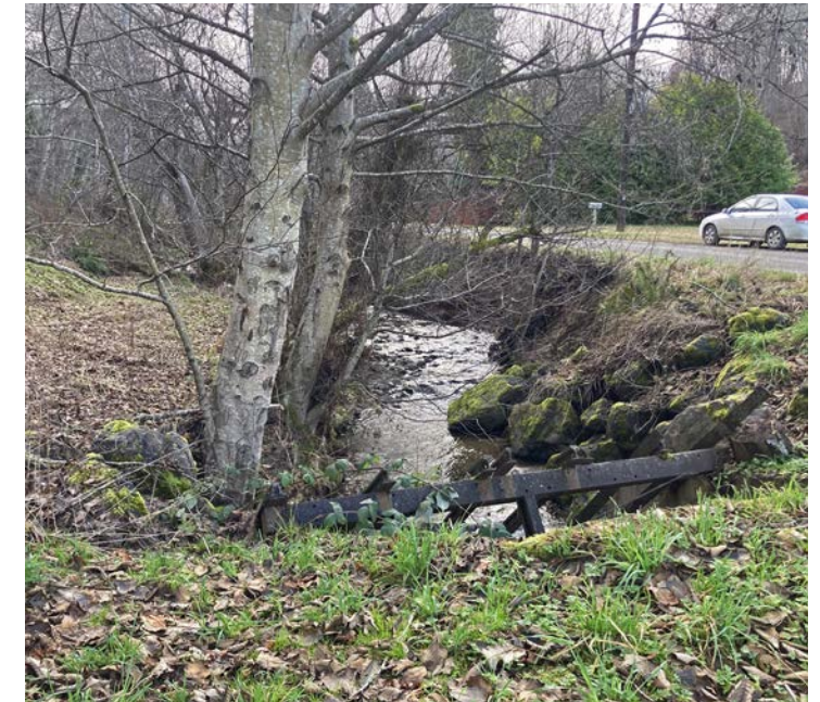
Figure 8. Riprap at inlet to Lower Valley Creek culvert system, adjacent to South Valley Street
