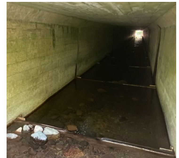
Figure 62. View of wooden baffles installed along the bottom of the Valley Creek culvert under Highway 101
