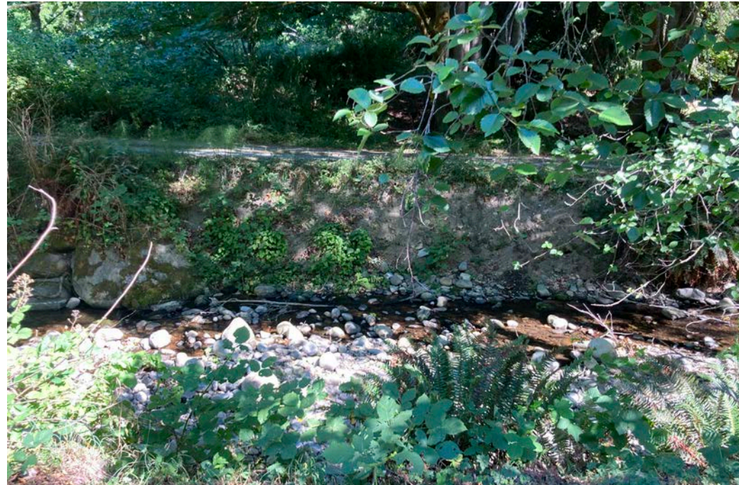
Figure 78. Road eroding into Valley Creek
