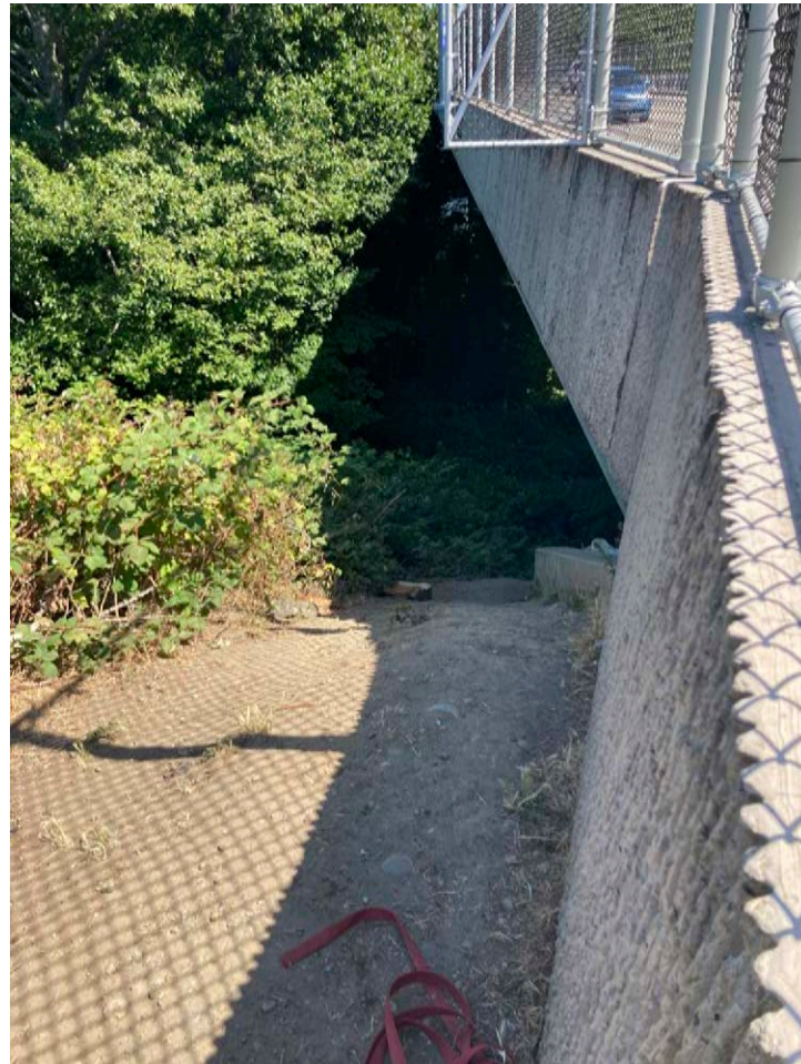
Figure 75. Erosion above Valley Creek at northeast corner of West 8th and South Pine
